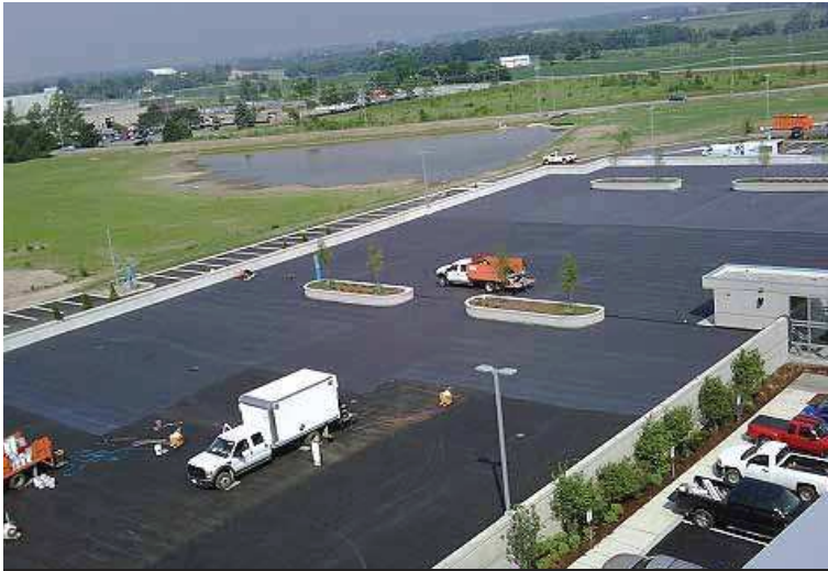
Waterloo, ON: Image of Project Installation at Research In Motion's Main Office Area
